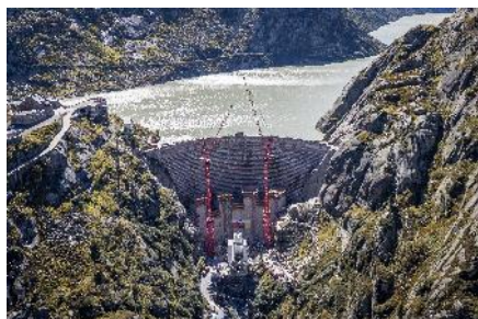
Kraftwerke Oberhasli AG Capacity: 1'232.0 MW End of the concession: 2042
