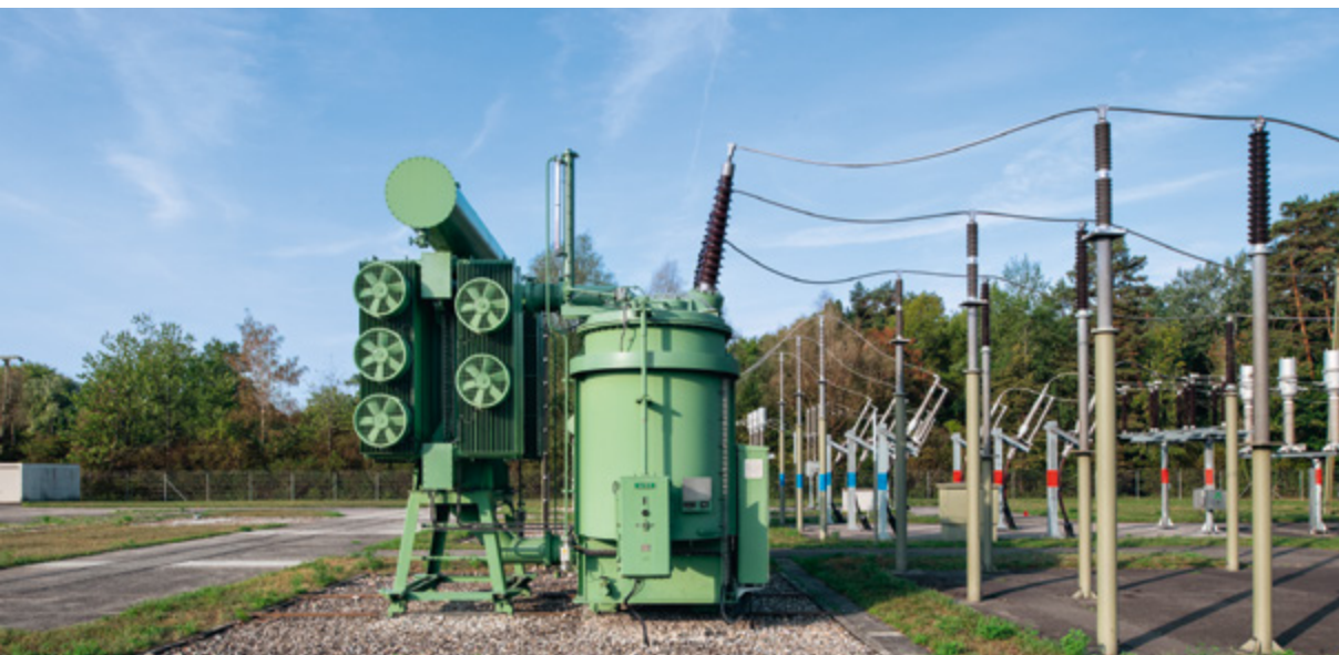
At BKW, transformers are reused whenever possible.
